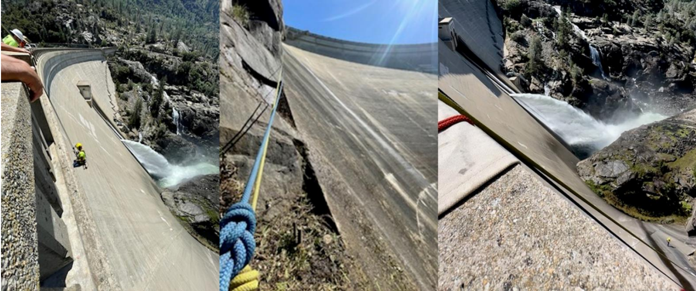
Hetch Hetchy Water and Power (HHWP) Maintenance Engineering staff inspect the face of O’Shaughnessy Dam. This inspection utilized the expertise of numerous HHWP work groups to safely collect valuable information about the condition of the dam.
