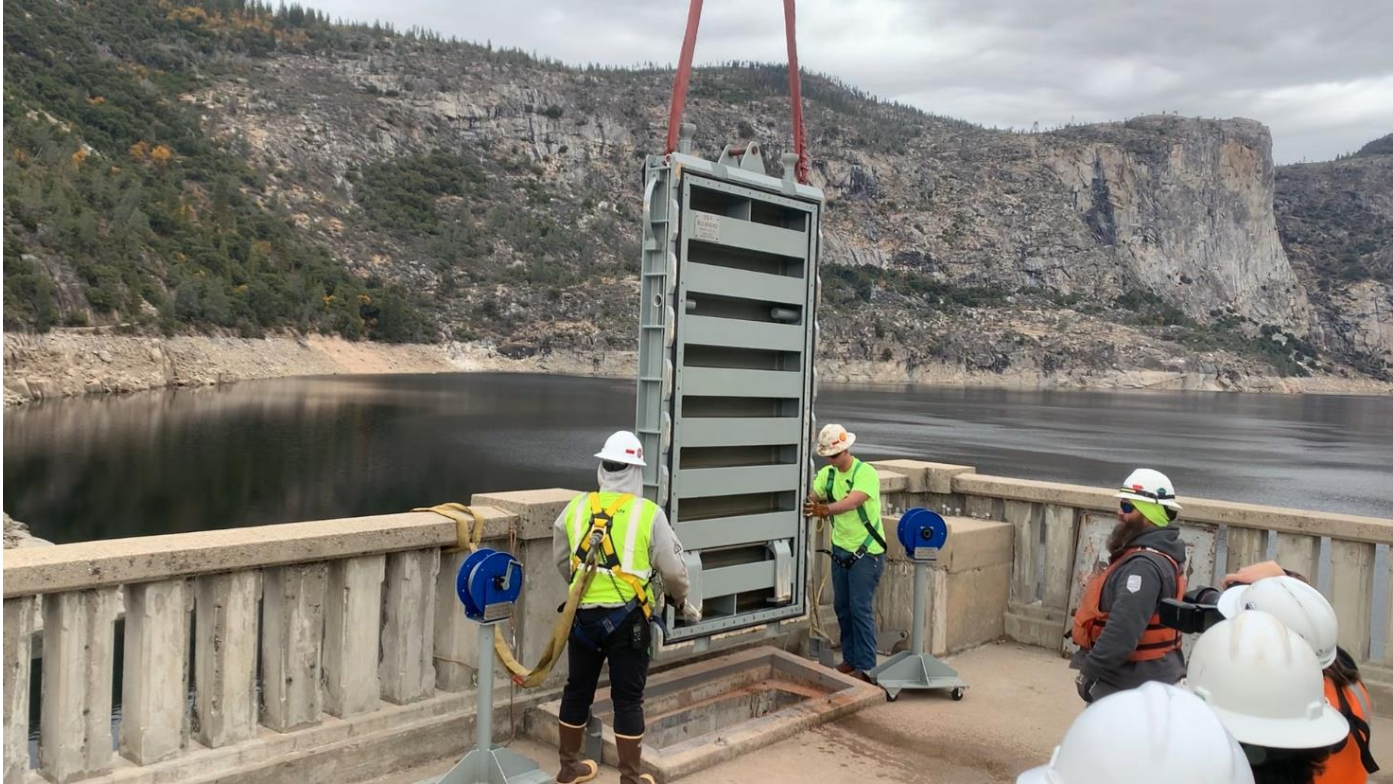
Hetch Hetchy Water and Power staff observe the test installation of a new bulkhead at O’Shaughnessy Dam. The new bulkheads will allow the SFPUC to work on future projects on O’Shaughnessy Dam appurtenances, including the face valves, slide gates and Canyon Tunnel.
