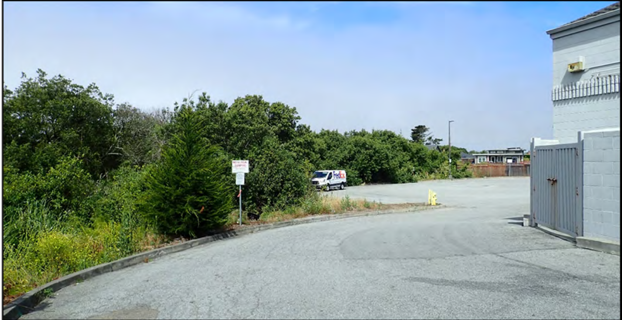
Photo 5a: Bore entry staging area (beyond fire hydrant) behind Safeway in the Strawflower Shopping Center.
