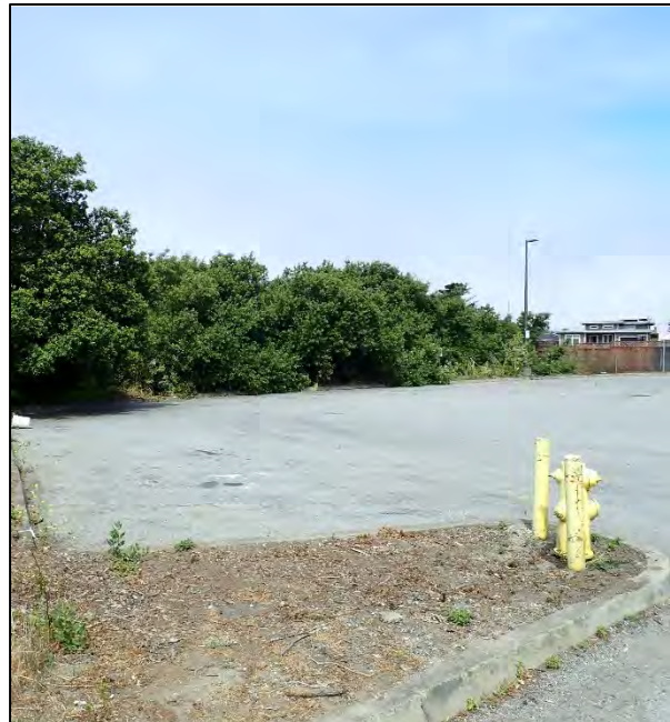
Photo 5c: Bore entry location and tie-in to existing water line (under Fire Hydrant).
