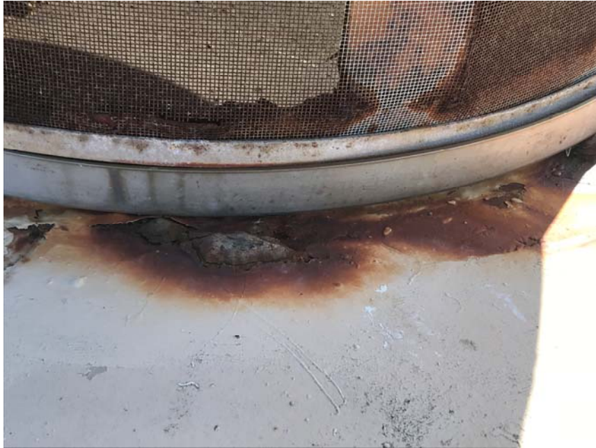
Photo 5: Corrosion around Perimeter of Roof Vent
