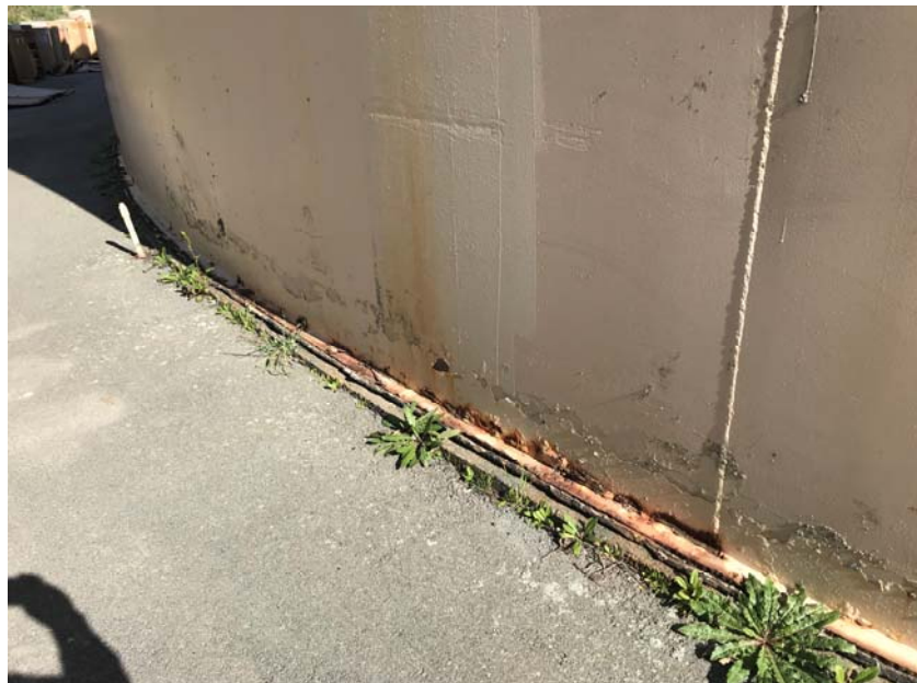
Photo 2: Corrosion on Tank Shell Plate
