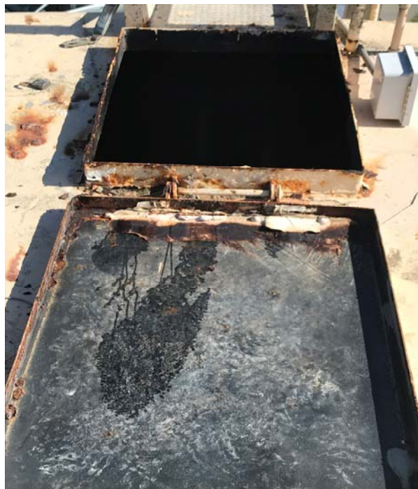
Photo 6: Corrosion on Roof Hatch
