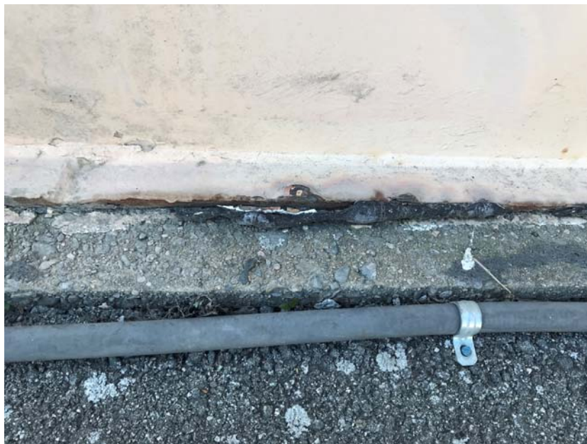
Photo 4: Degraded Caulking along Perimeter of Bottom Plate
