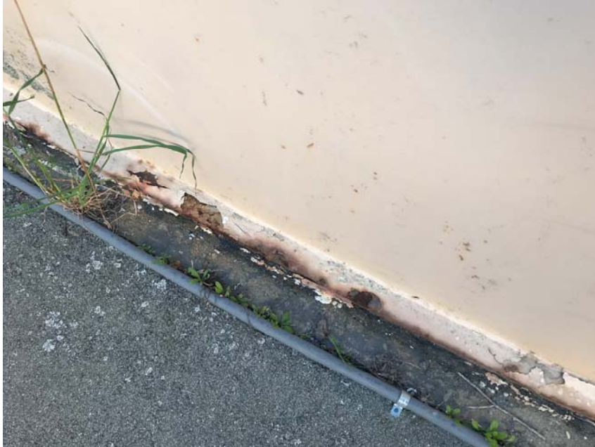
Photo 1: Corroded Tank Bottom Plate
