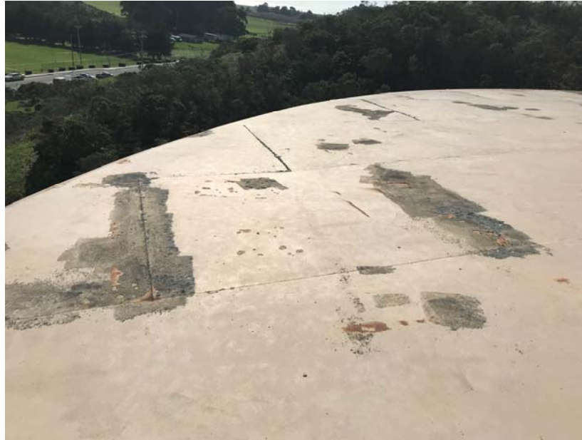
Photo 3: Corrosion on Tank Roof Plate
