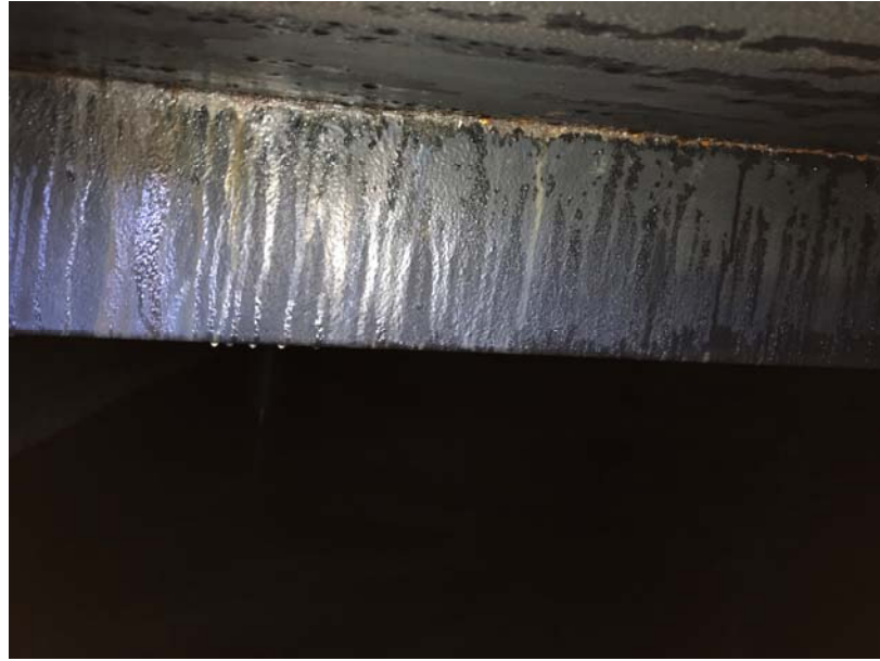
Photo 7: Condition of Existing Exterior Rafters
