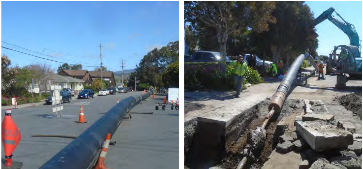
Figure 3 – Example of pre-fabricated product pipe string [Left]; Pullback of product pipe [Right]
