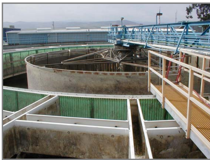
View of John Jones Water Treatment Plant primary clarifiers
