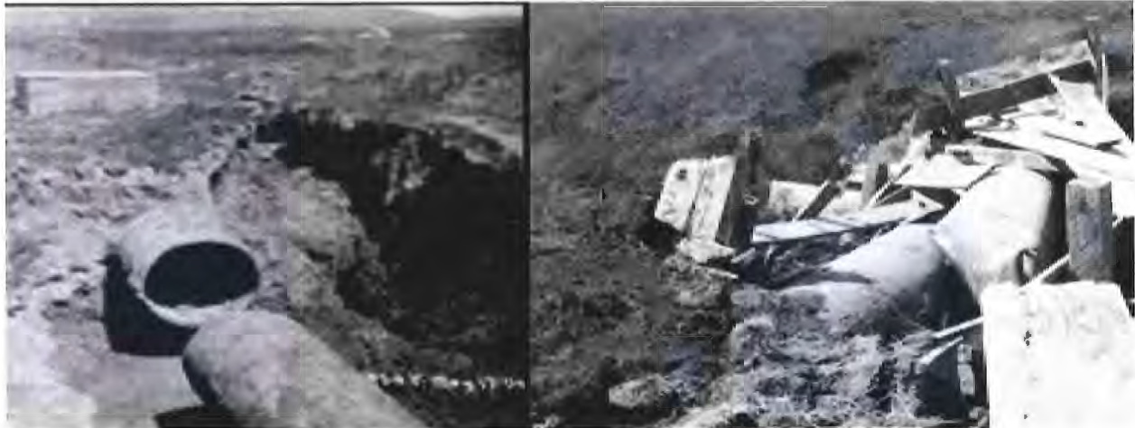
Figure 2: Water Mains Damaged by the 1906 San Francisco Earthquake
