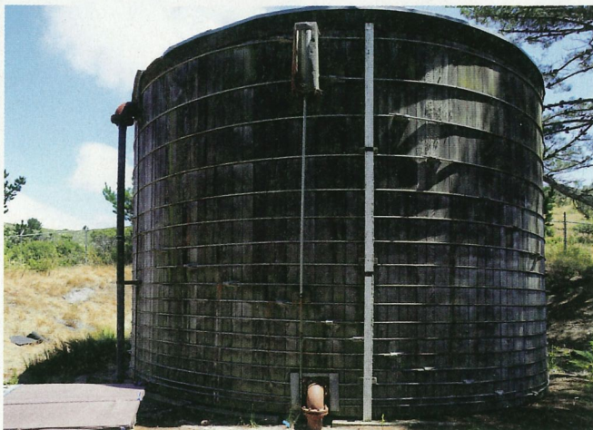
Original Hazens Tank made of redwood
