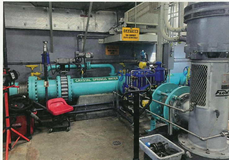
Crystal Springs Pump Station
