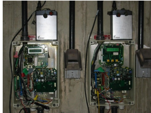
Figure 5: 4-20mA Signal Data Logging
