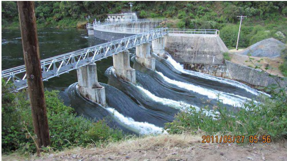
Early Intake Reservoir & Diversion Dam – Early Intake reservoir was constructed in 1924 on the Tuolumne River 17 miles below O'Shaughnessy Dam. The structure's purpose was to divert water into Mountain Tunnel and to Moccasin Powerhouse as water made its journey to the Bay Area. About 8,400 cfs is shown here. (M. Patterson)
