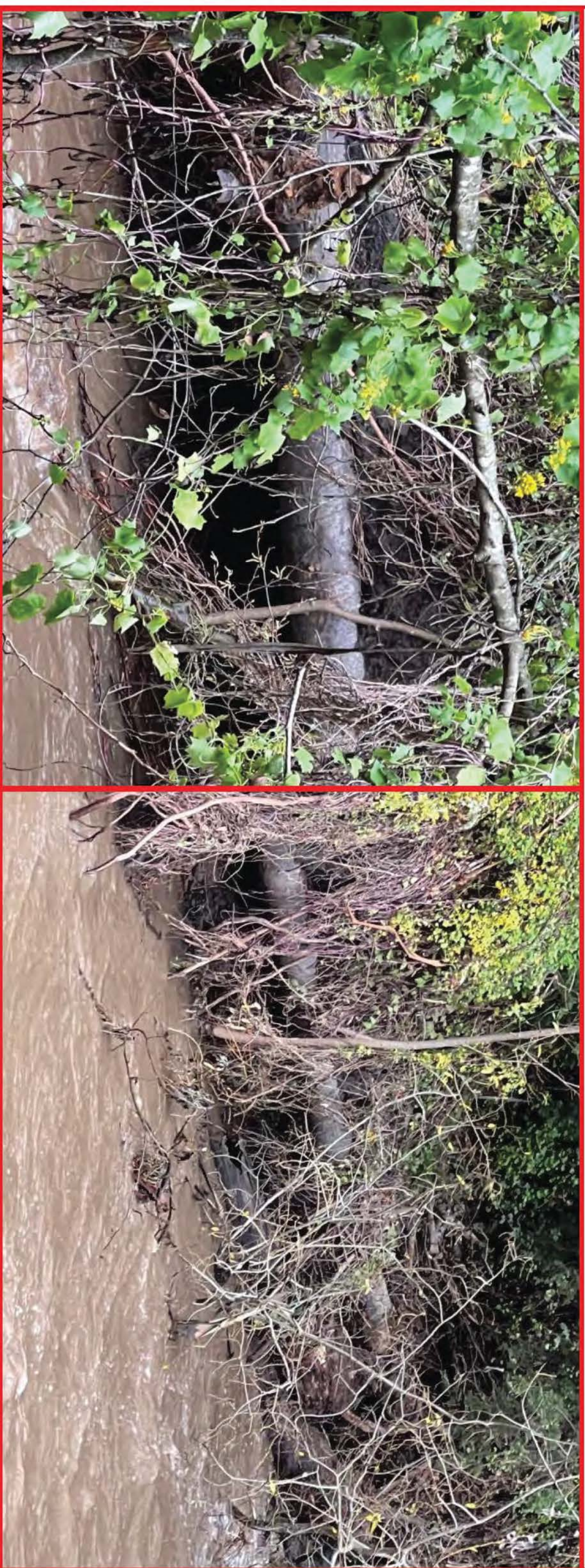
PIPE EXPOSURE AND DAMAGE CAUSED BY THE JANUARY 2023 WINTER STORM DISASTER.
