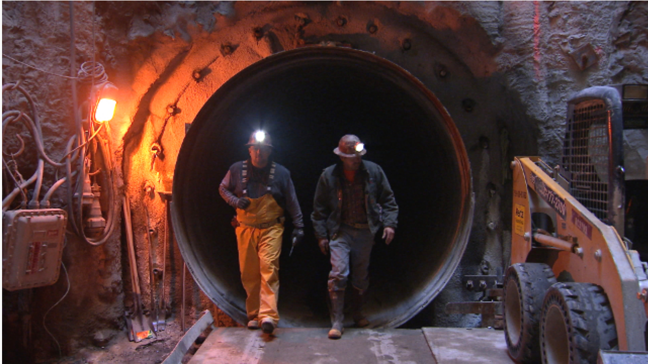
Workers with the San Francisco Public Utilities Commission inspect the New Irvington Tunnel, which will carry an average of 265 million gallons of water a day. (Owen Bissell/KQED)
