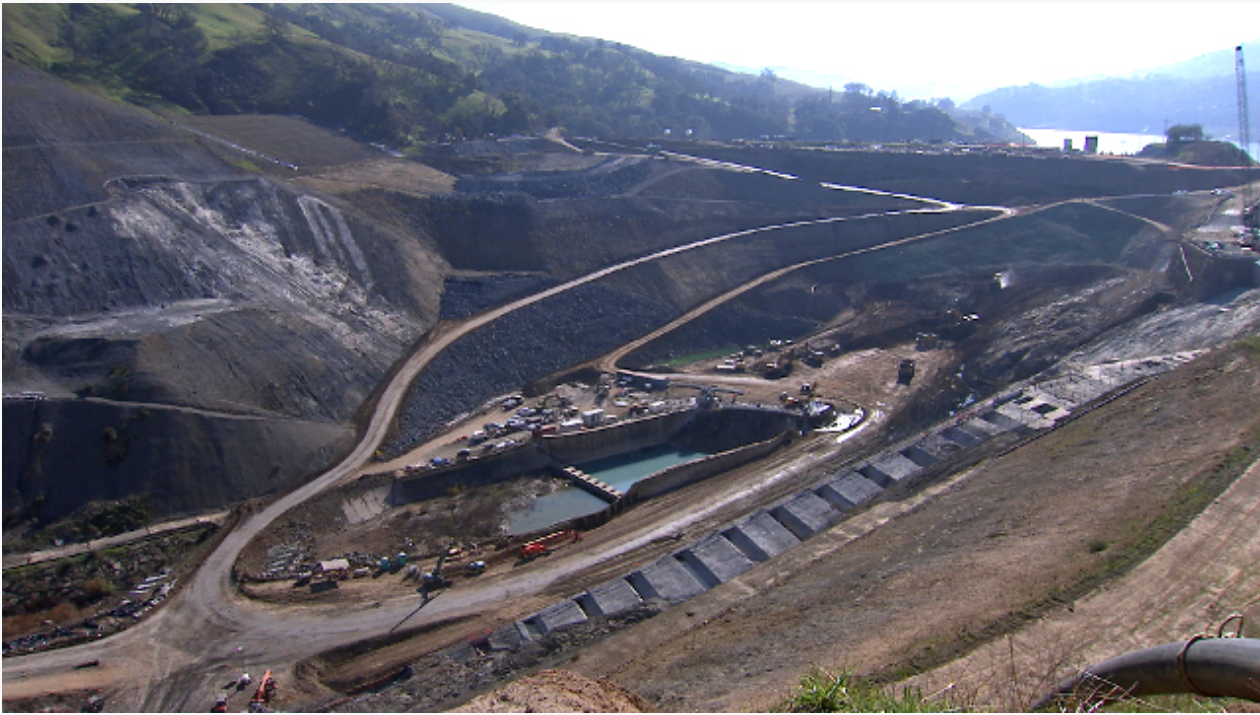
Ten million cubic yards of earth and rock will need to be excavated for the construction of the new Calaveras Dam, located at the Alameda-Santa Clara county line. (Owen Bissell/KQED)
