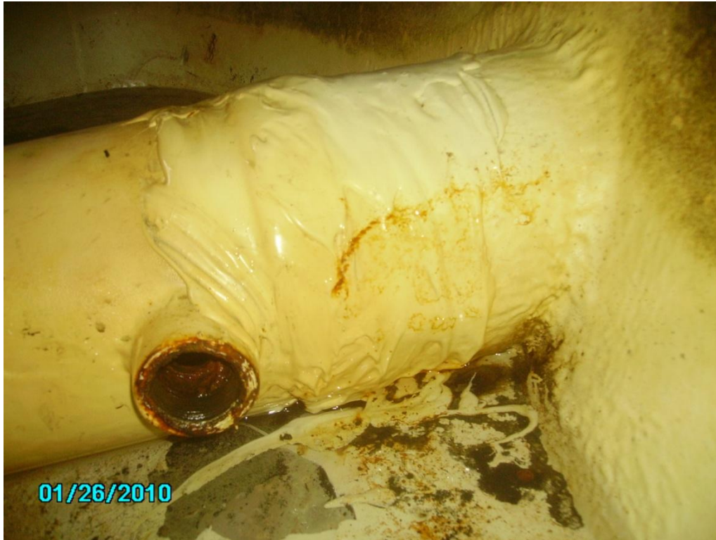
Photo 4. Location of Crack in Filter 1 Manifold Pipe
