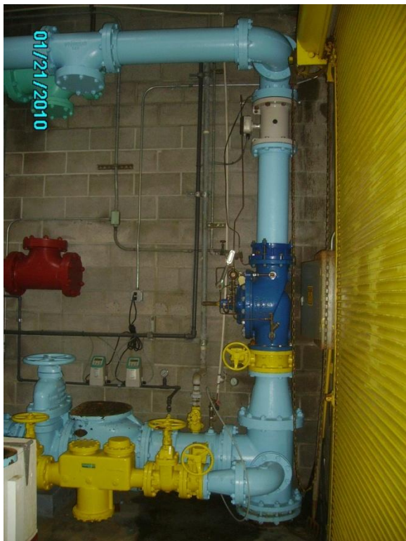
Photo 6. Filter Effluent and Backwash Supply Piping
