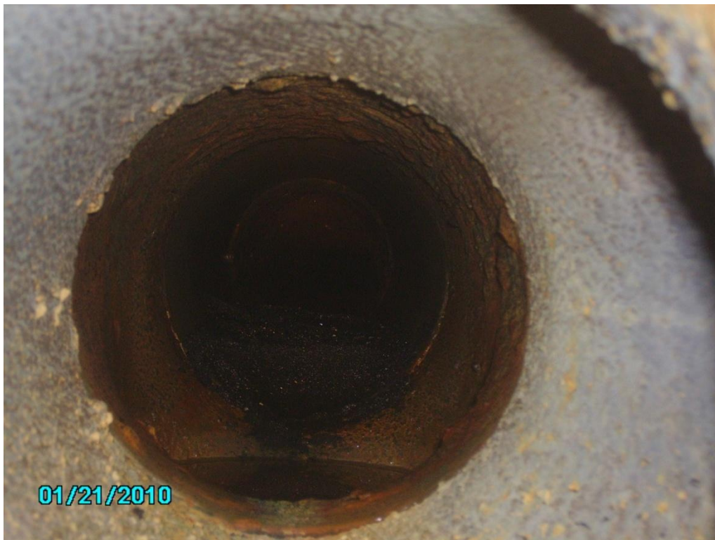
Photo 3. Filter Media Inside Filter Underdrain Manifold Pipe
